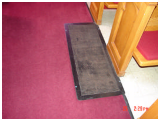
Picture 20- Supply air grill
