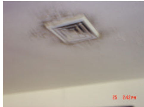
Picture 38- Nursery 12 Ceiling
