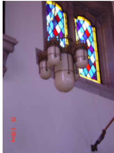
Picture 36- Nave Light Fixtures
