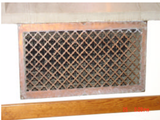
Picture 19- Return Air grill
